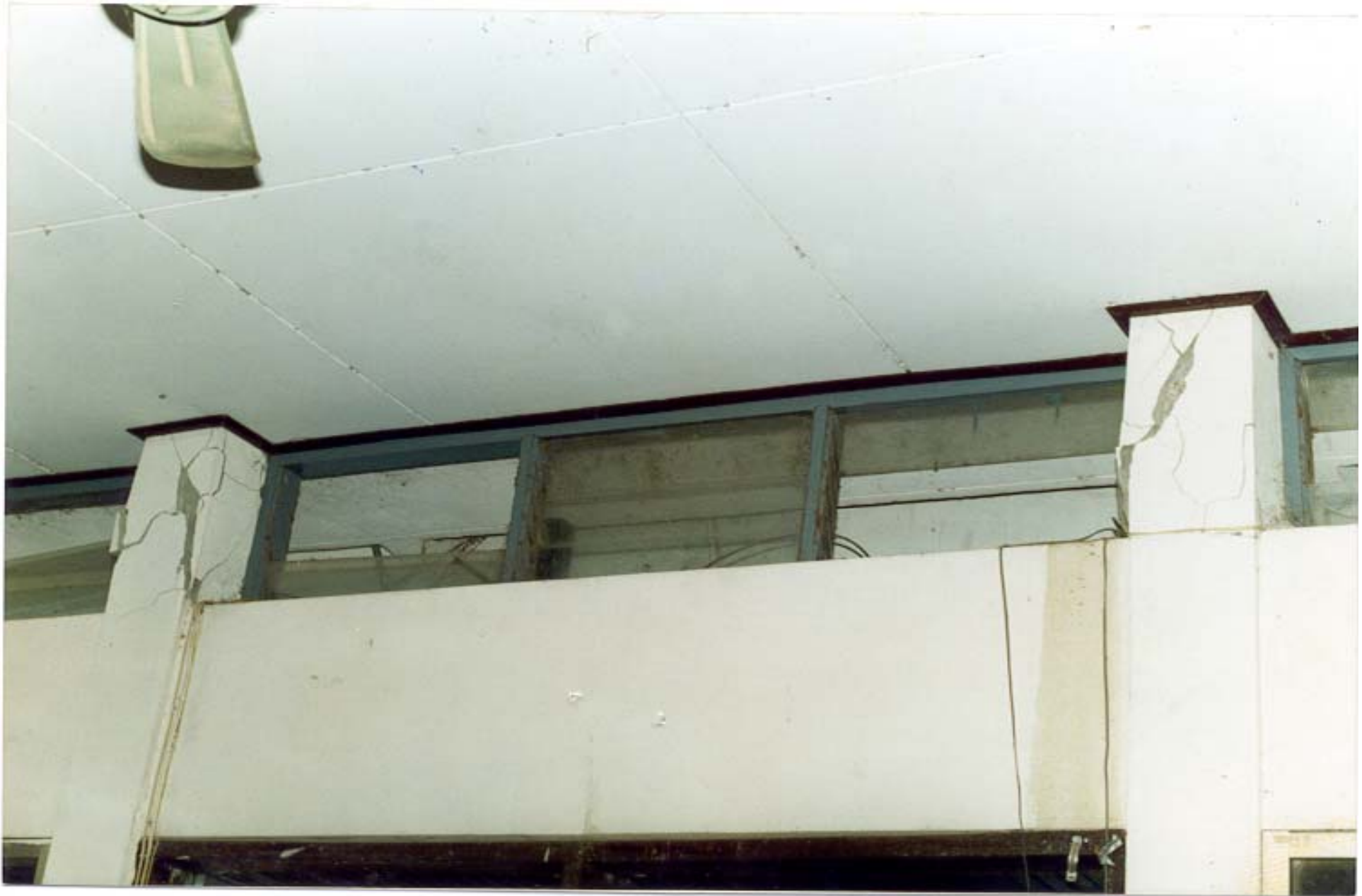
Shear failure in short columns observed even in moderate earthquake
