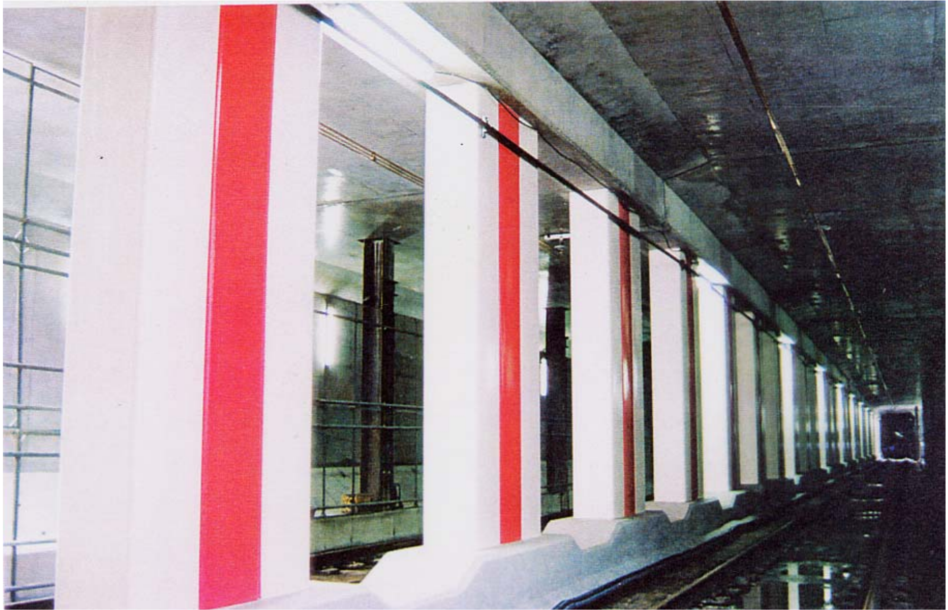
View of reconstructed B2 floor of Daikai Station, center pillars made by composite structures of steel box and RC.
